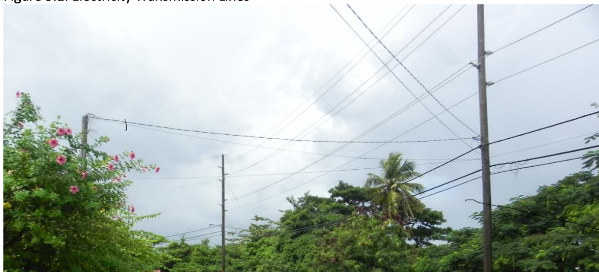
Figure 5.1: Electricity Transmission Lines
